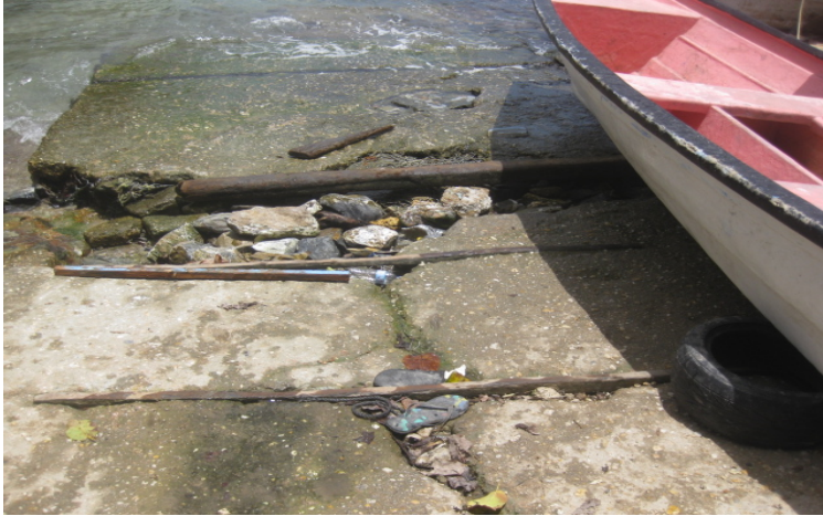
Figure 4.1: Defective ramp at the Blanchisseuse Fishing Facility.
