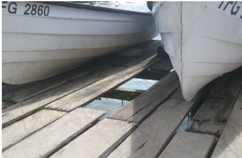
Figure 4.3: Missing planks on the surface of the jetty at the Blanchisseuse Fishing Facility.
